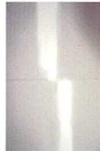
Finished butt joints! Left is on stud and right in between studs
