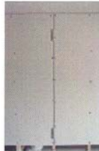
Install 2nd board and remove the Space Bars
